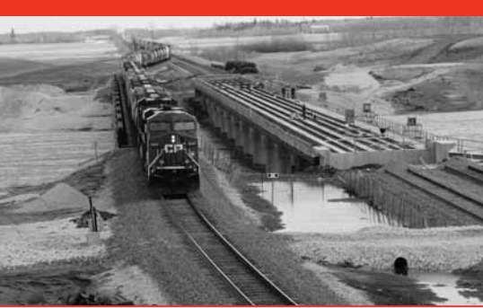
A detour structure reroutes trains while work on CP Keewatin Bridge is underway.
