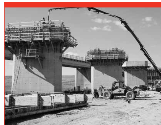
Work on the CP Emerson Bridge is scheduled for completion in fall 2009.
